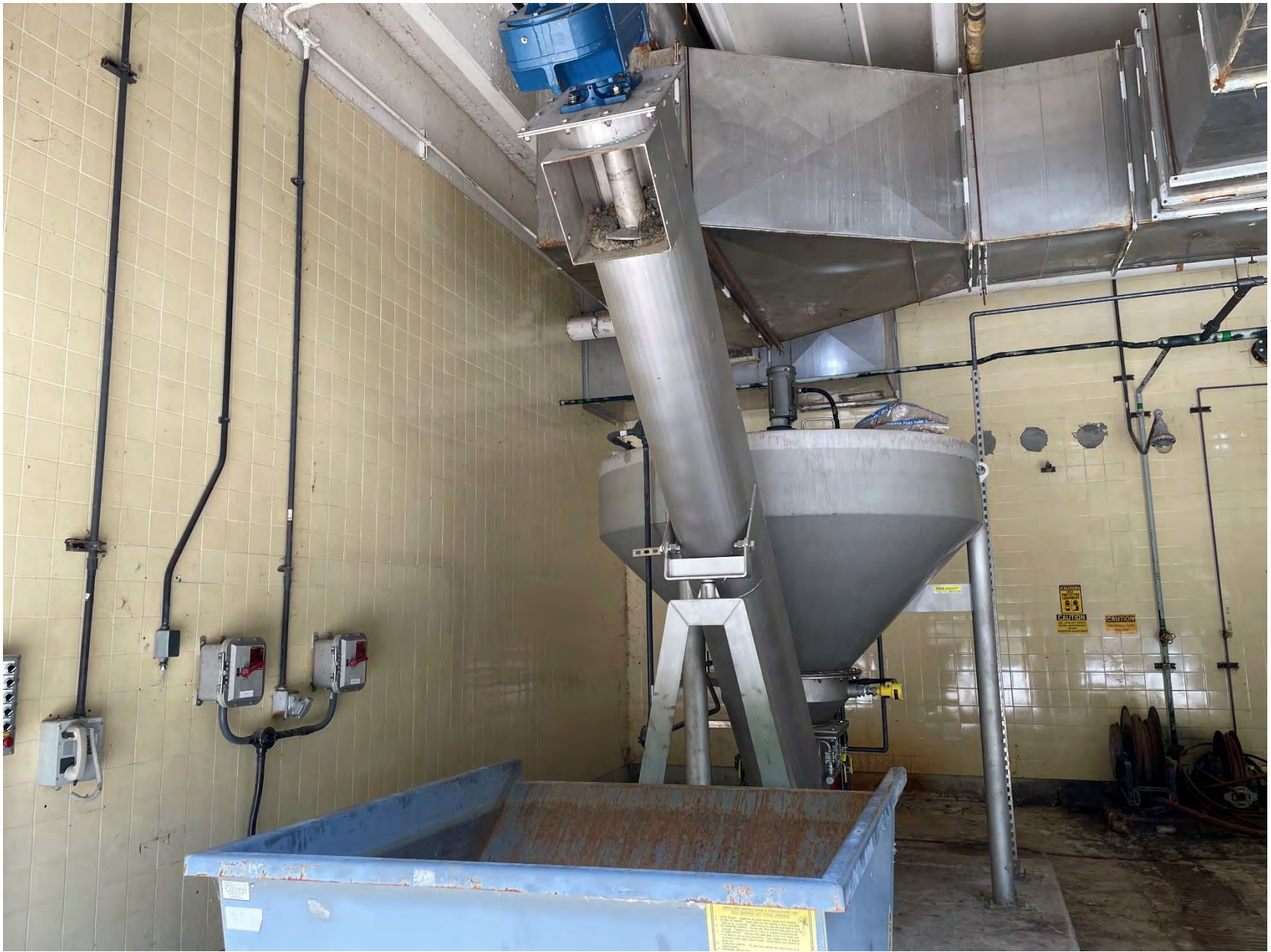
Photo 6- New Grit Cleanser processing grit.
