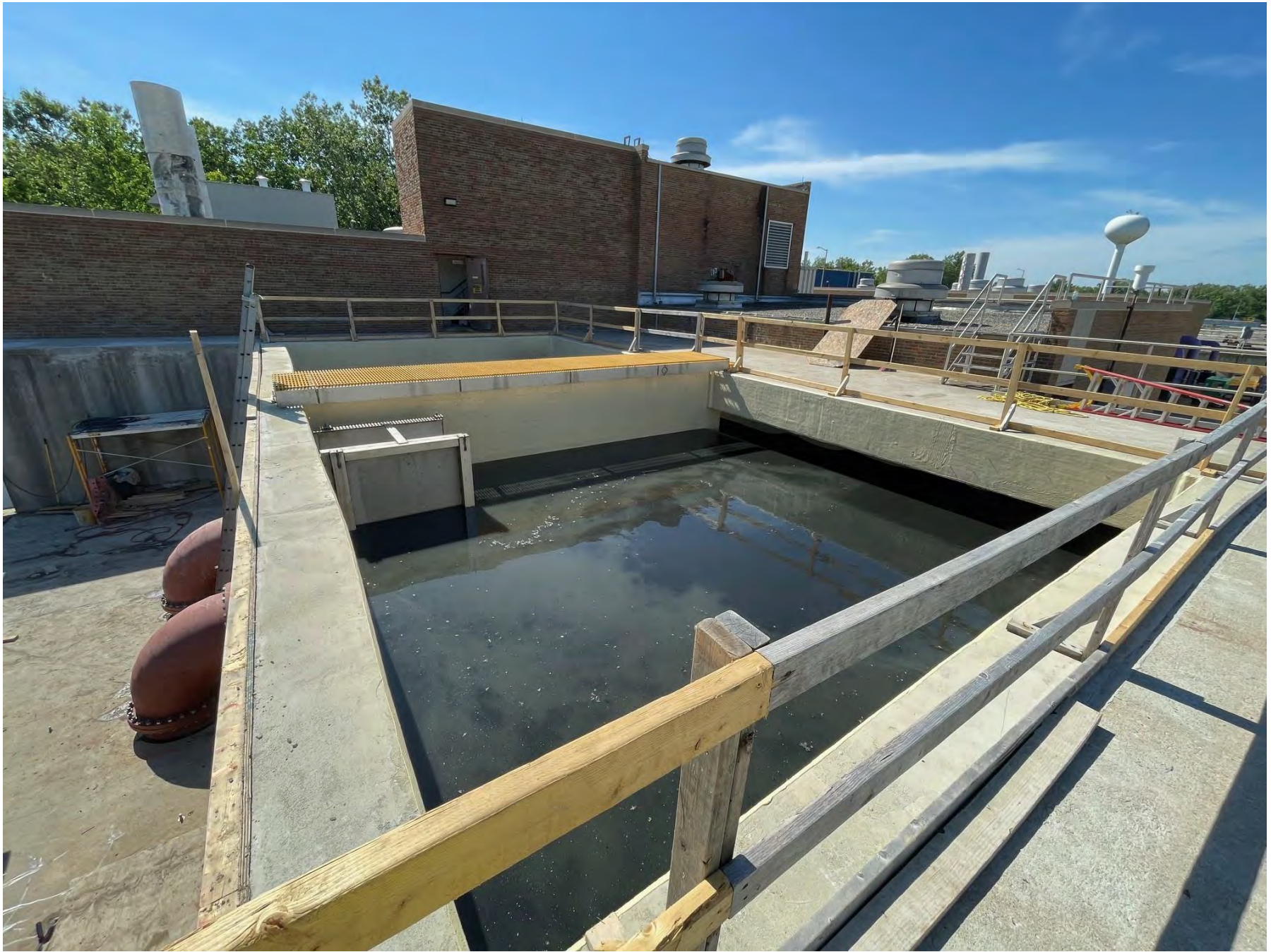
Photo 5 – East Grit Tank operating and flow spilling into Grit Channel.
