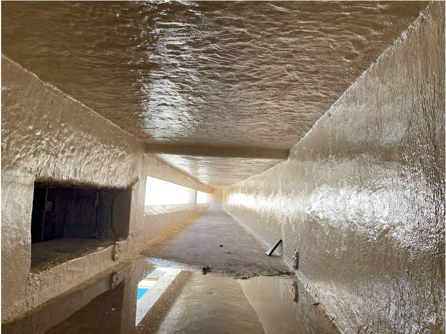
Photo 1 – Grit Channel with Type 9B Coating
