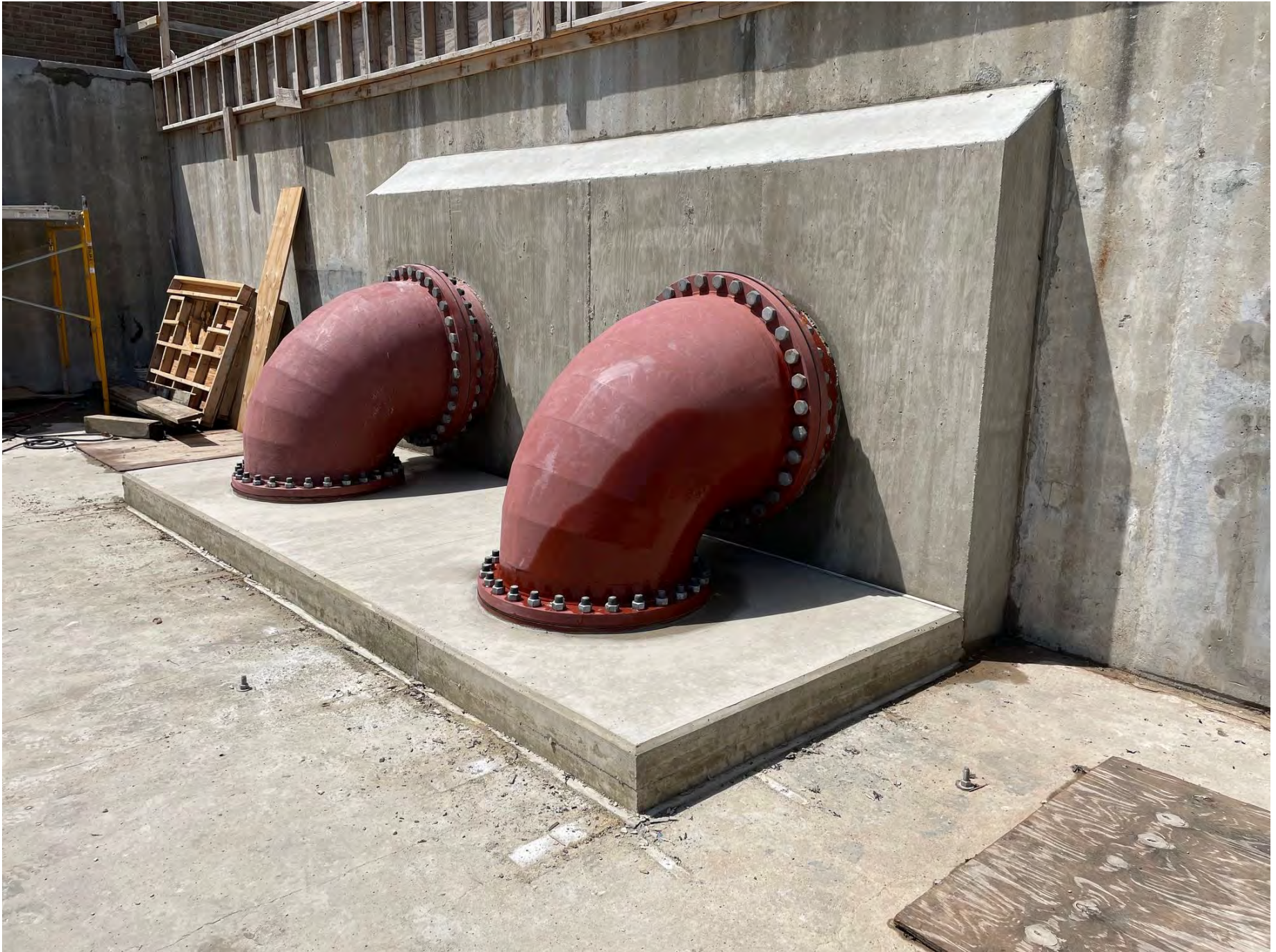
Photo 2 – New grit influent piping and concrete collars leading from influent pumps up into Grit Tanks.
