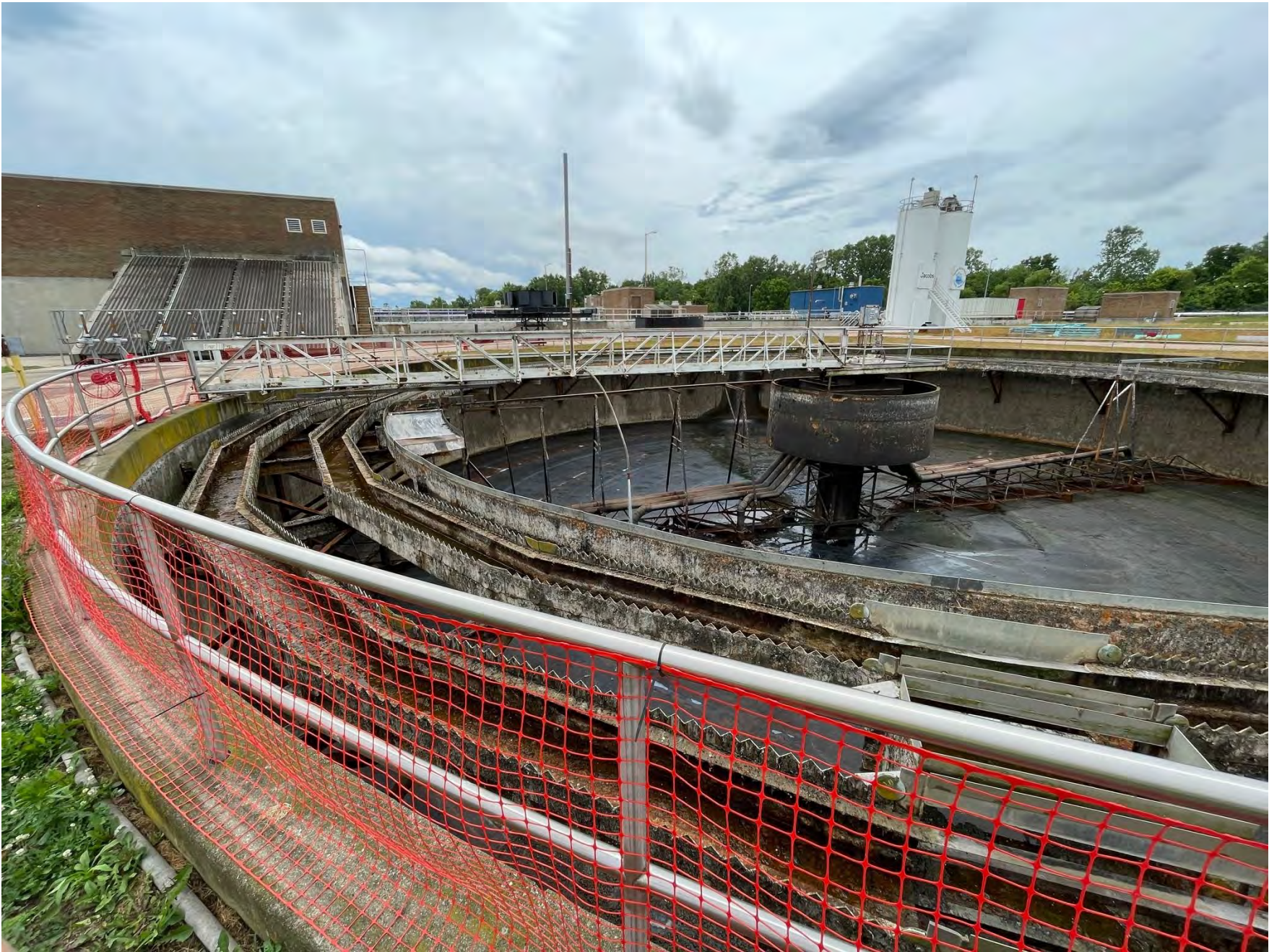
Photo 7 – Final Clarifier 2 drained and ready to start demo. Final Clarifier 4 was started June 27 th successfully demonstrated.
