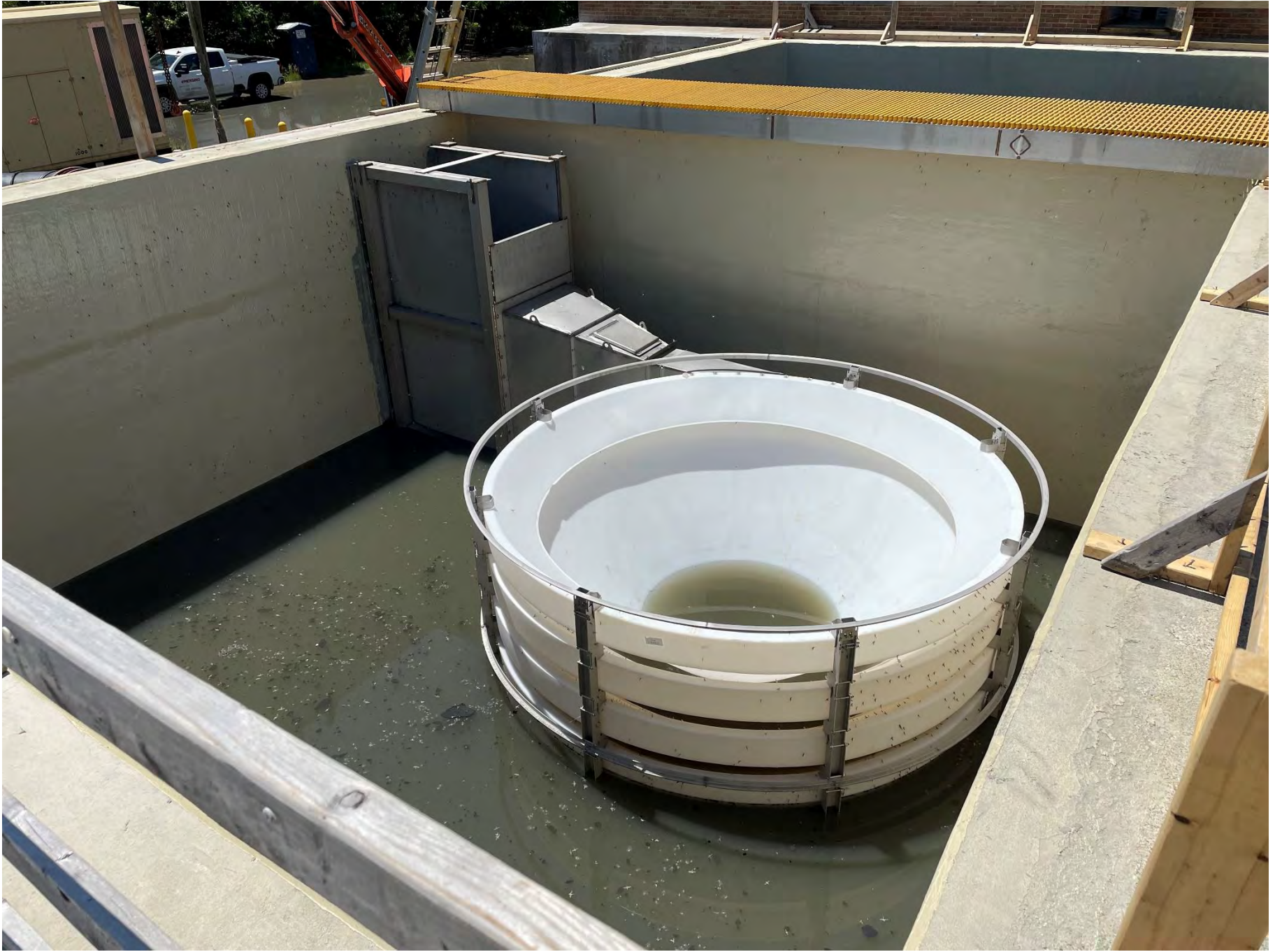
Photo 3 – East Grit Tank during startup. Stack tray and transition channel visible prior to fulling filling.
